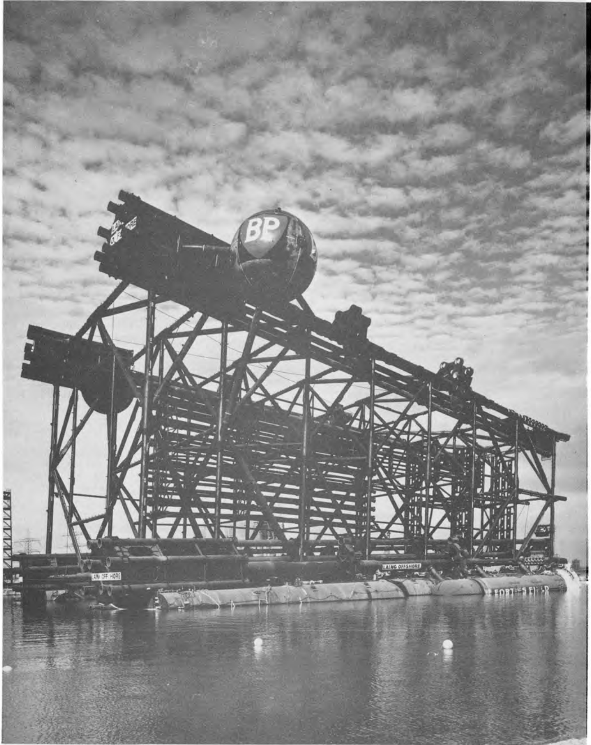
Fig.1. The BP Forties FB platform leaving Greythorpe yard in the horizontal position prior to its rotation and erection offshore. (Photograph: John Laing and Sons Ltd)
